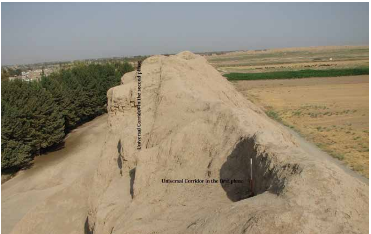
Fig.5. The first and second phases of corridors within the defensive wall of Qaleh Iraj. The second phase of the corridor was filled with bricks during the third phase. Source: authors' archive.
