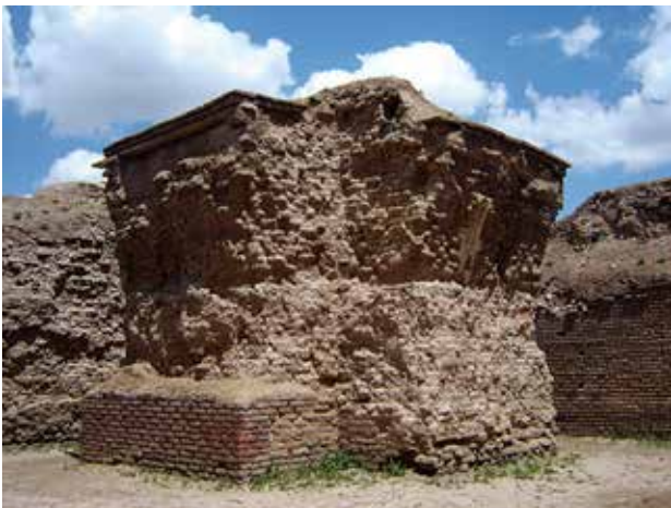
Fig. 10. One of the wall-columns of the Azargoshansb Char-tagh (the Fire Place), Takht-e Soleiman World Heritage Site, West Azerbaijan. Photo: Keyhanpoor, 2005.
